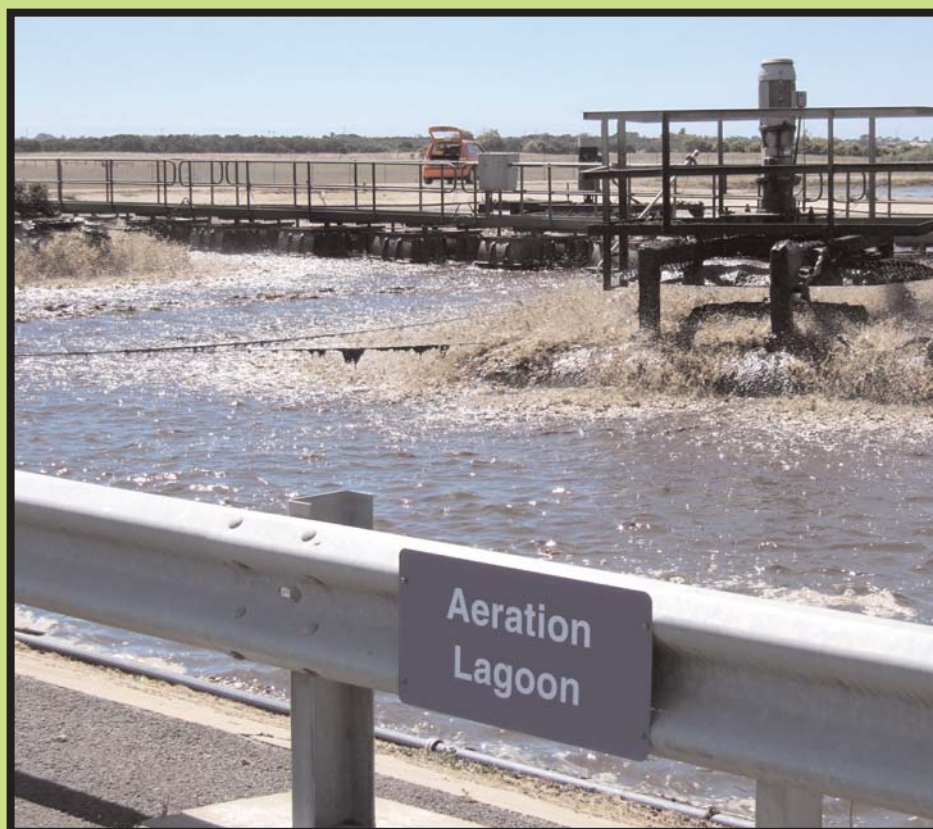
Figure 1: Aeration stage of sewage treatment. Photo by David Wang, courtesy of South East Water Ltd., Melbourne.
